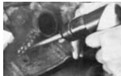
This photo shows a repair with plugs installed and peened ready for resurfacing the casting.
